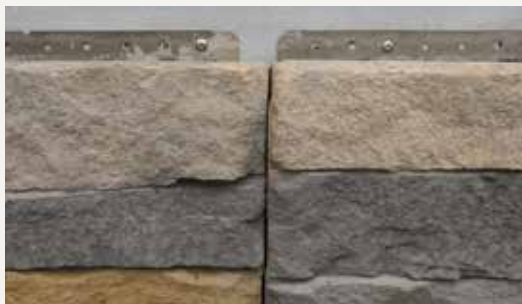
Poor choice of mating panels. Panel stone sizes are too similar from panel-to-panel.
