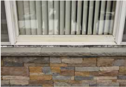
Three sills required on this window. Center and cut middle sill to avoid cut ends on end (most visible) sills.
