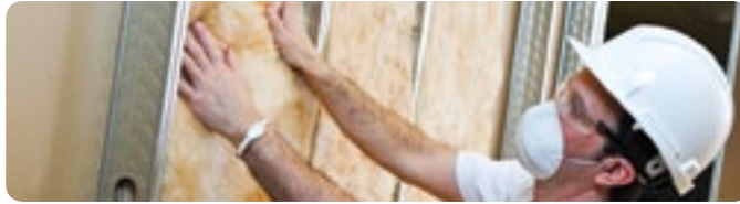
CertaPro™ Commercial Insulation
